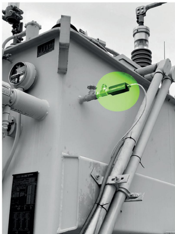
Figure 1. Hydrogen sensor (in green) mounted to an electricity transformer.
