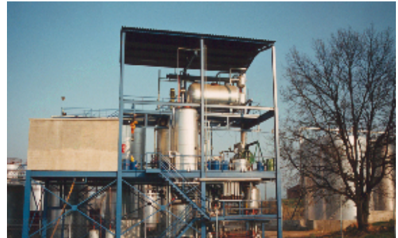
Figure 1: Partial hydrogenation unit
