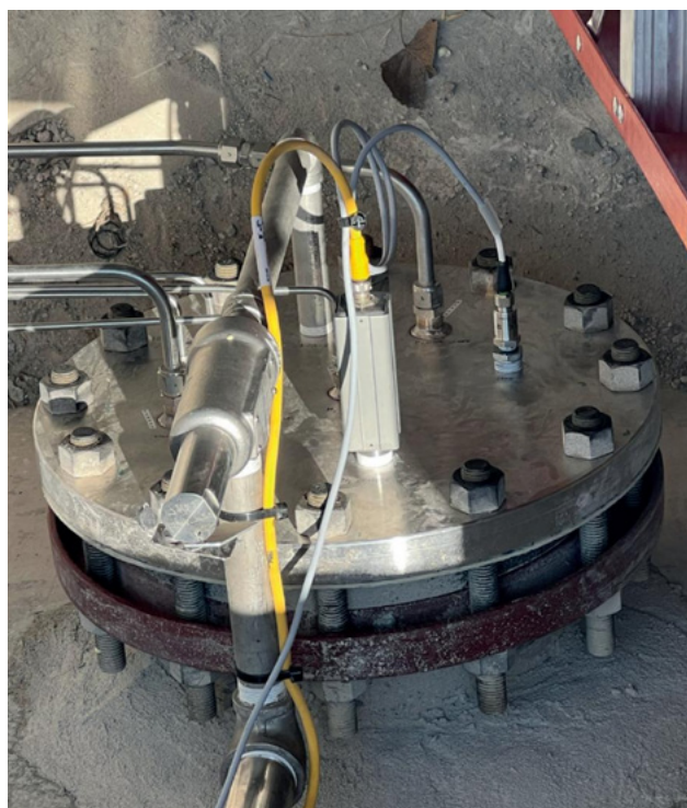
Figure 1. A flange connected to the H2C Safety Pipe test system. Pressurised hydrogen fills an inner carrier pipe made of fibreglass-reinforced polymer. An outer 'safety' pipe contains any leaks; and the H2scan sensor (the grey rectangular component connected through the flange into the space between the two pipes) measures hydrogen concentration within the annulus in real time.
